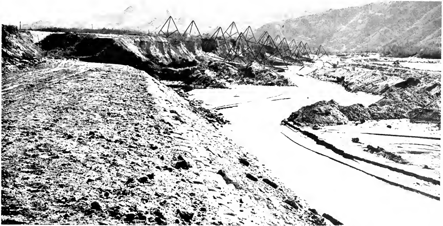
Thirty-foot steel rail tetrahedrons, shown in middle ground, and sacked concrete riprap installation in foreground
